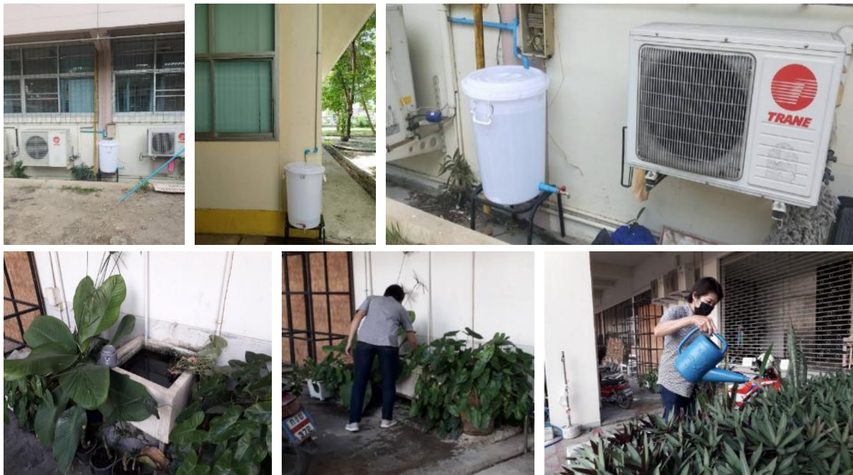
Water collection from air conditioning systems
