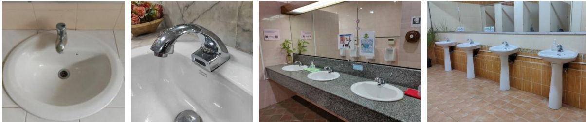
Low flow taps and automatic taps
