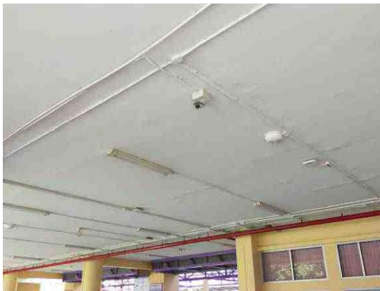
CCTV cameras in the building
