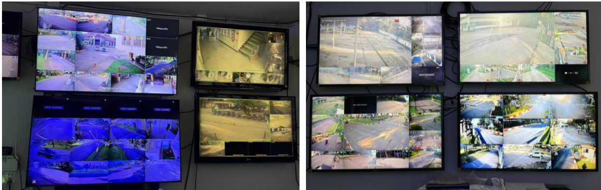
The university CCTV system control room
