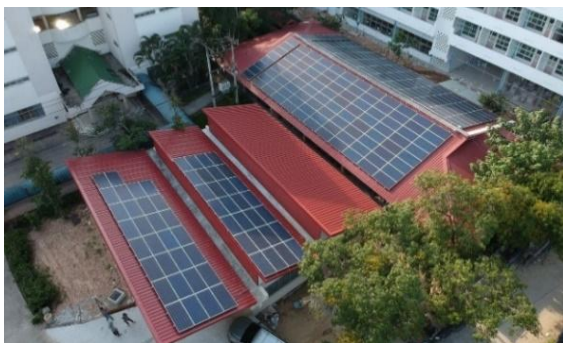
Solar rooftop with 80-kW installed capacity
