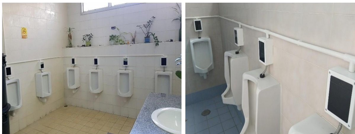
Smart urinal water-saving devices
