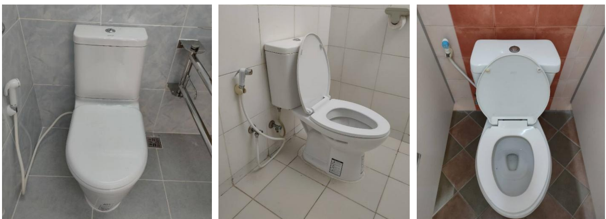
Low flush tank toilet
