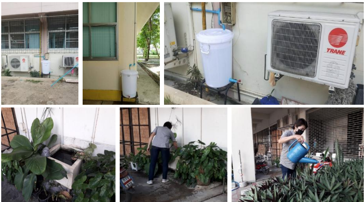
Water collection from air conditioning systems
