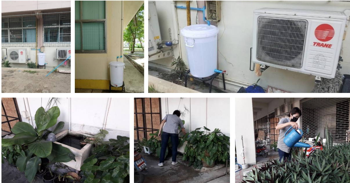
Water collection from air conditioning systems
