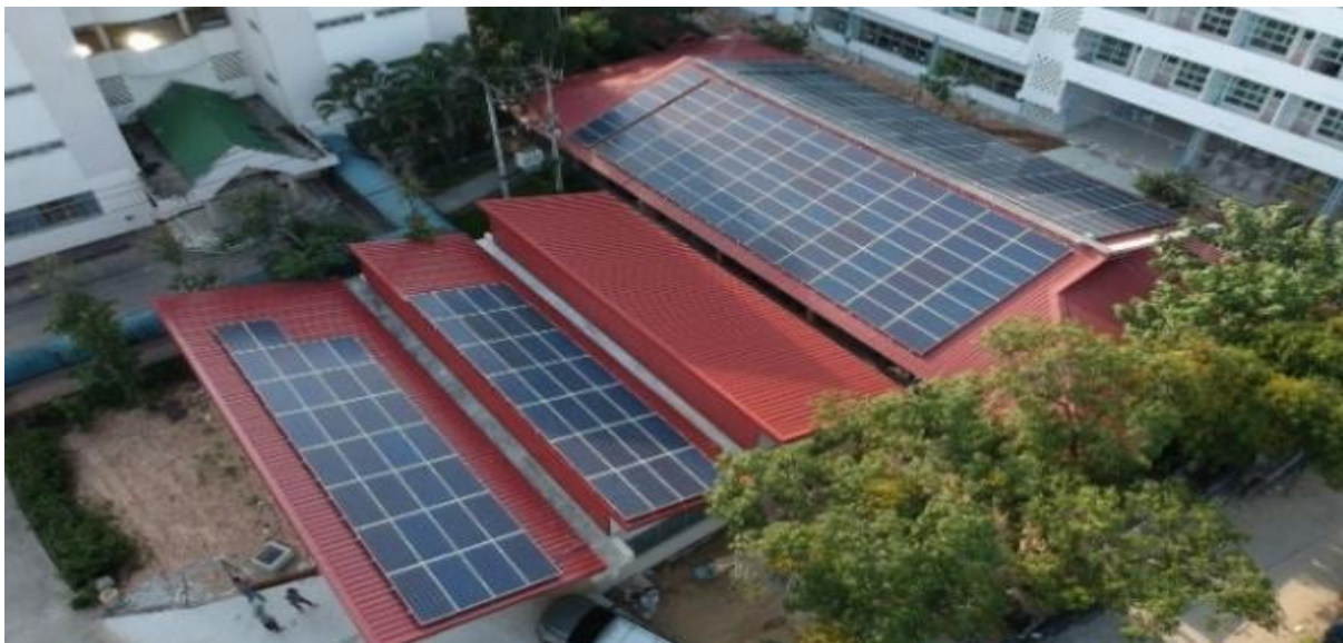
Solar rooftop with 80-kW installed capacity
