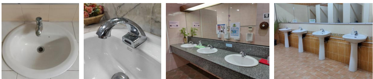
Low flow taps and automatic taps
