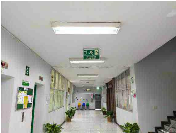
Fire exit sign
