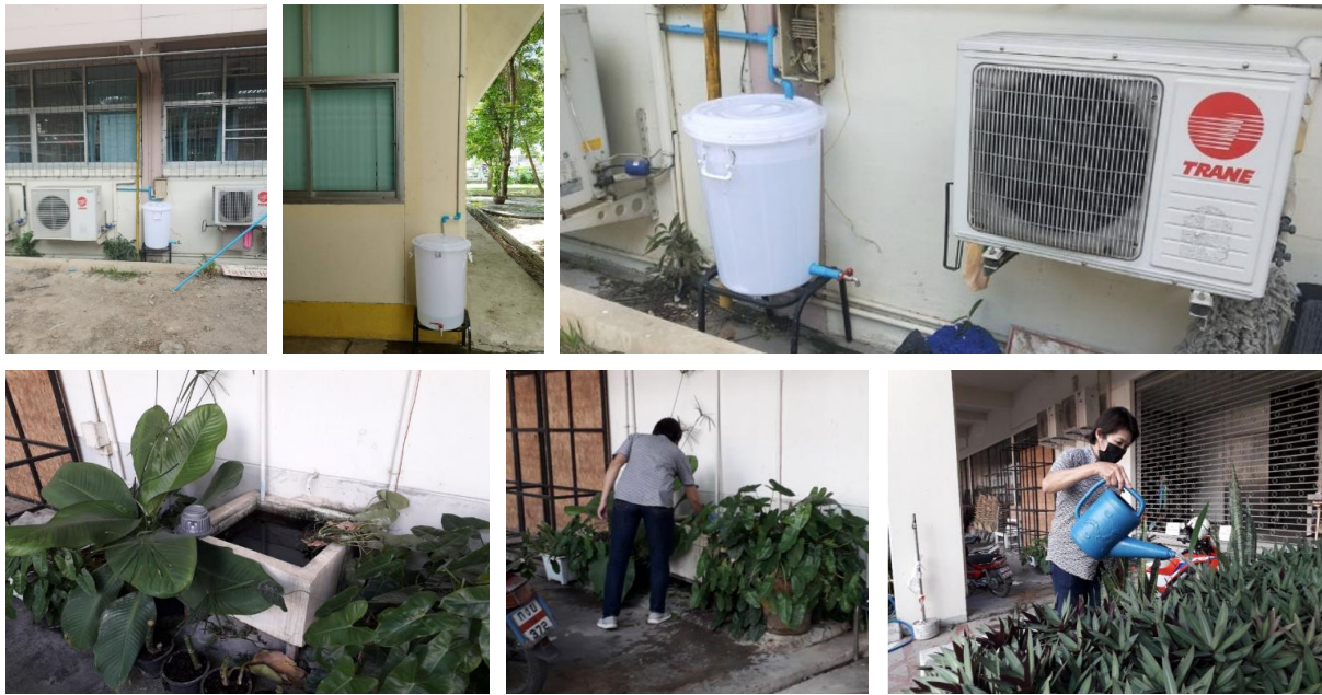
Water collection from air conditioning systems
