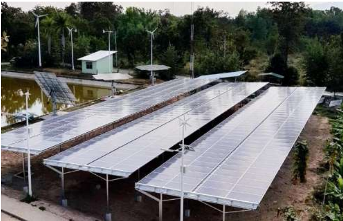
Scope 2: Purchased electricity from Solar PV module at solar rooftop of MJU
