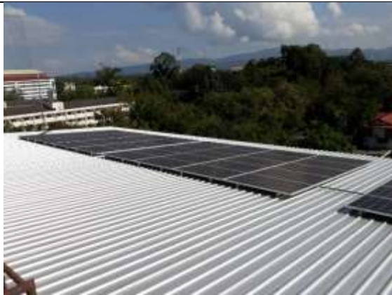
Solar rooftop station 1 capacity electricity of 20 kW
