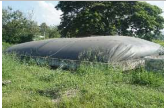
Biogas production system capacity of 300 m 3 for electricity
