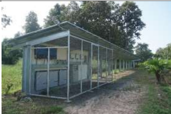
Solar rooftop station 3 capacity electricity of 40 kW
