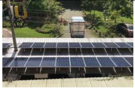
Solar rooftop station 6 capacity electricity of 20 kW
