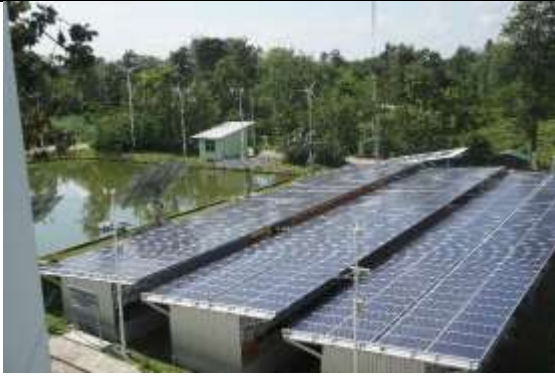
Solar rooftop station 5 capacity electricity of 300 kW
