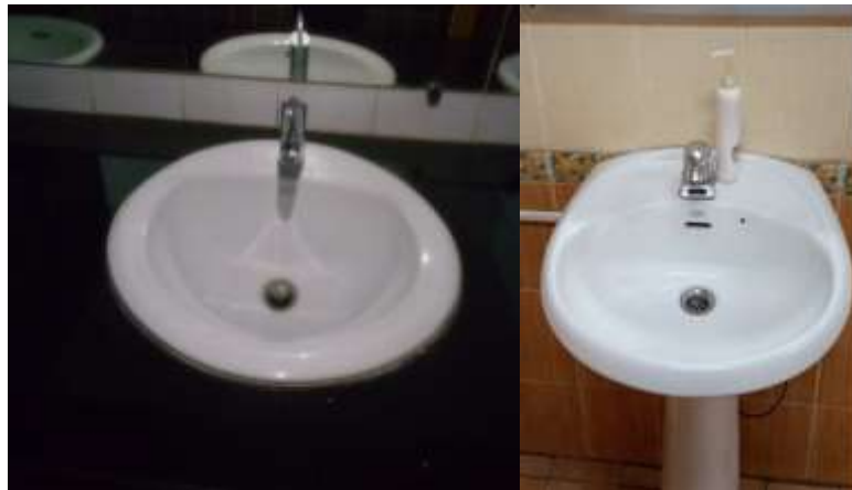
Washbasins water-saving push taps
