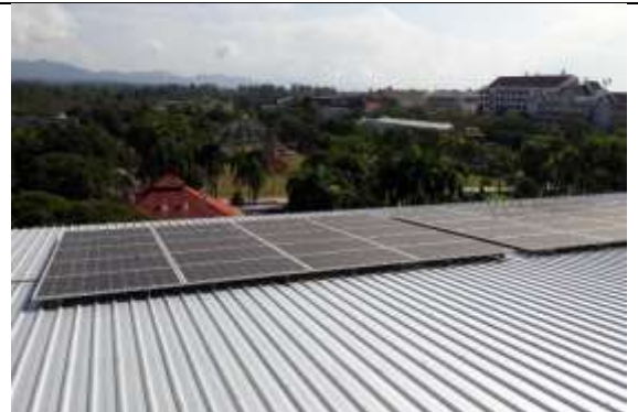
Solar rooftop station 4 capacity electricity of 90 kW
