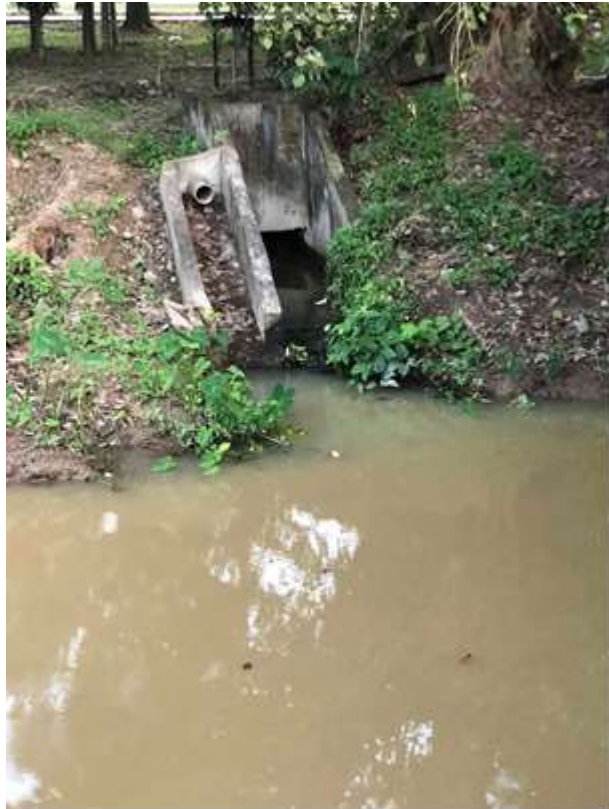
Treated wastewater released to the natural canal
